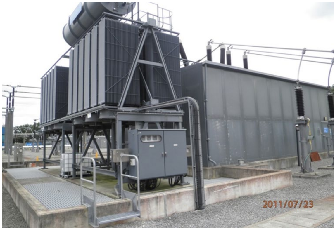
Image 4.5 Typical (large 400kV power transformer)
