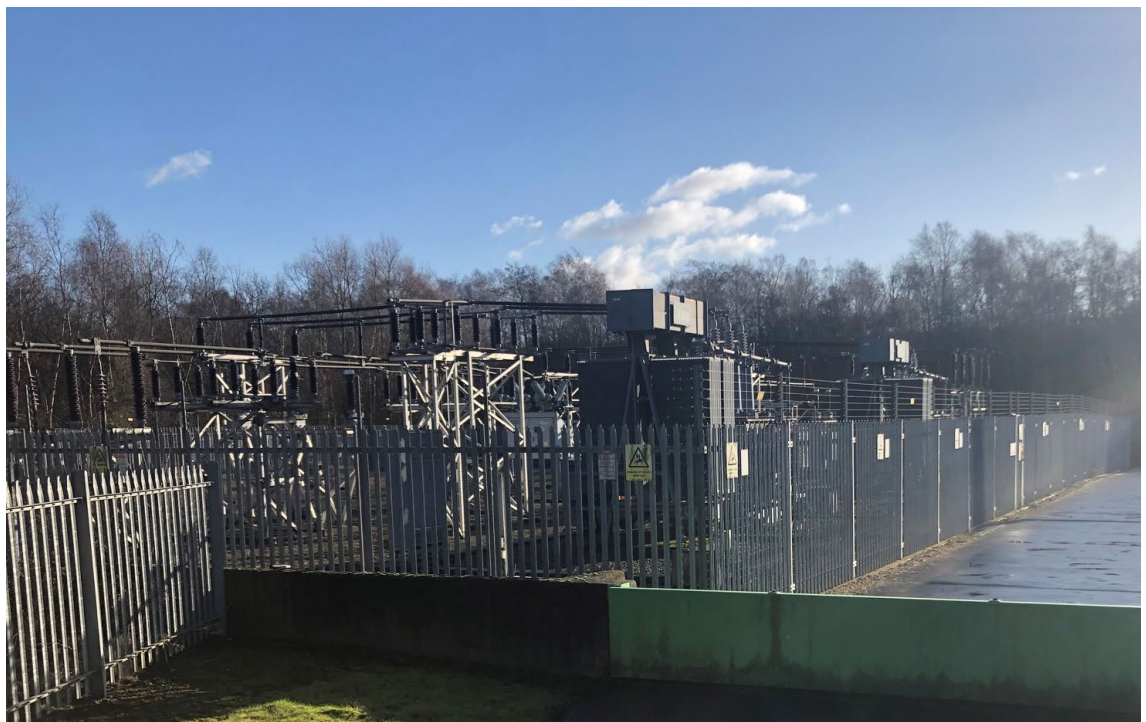
Image 4.6 Typical 132kV substation compound
